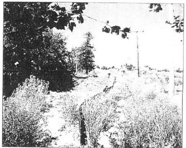
PHOTO 10: End of Labath Avenue facing north. Photo shows road construction on Lagner Avenue.
